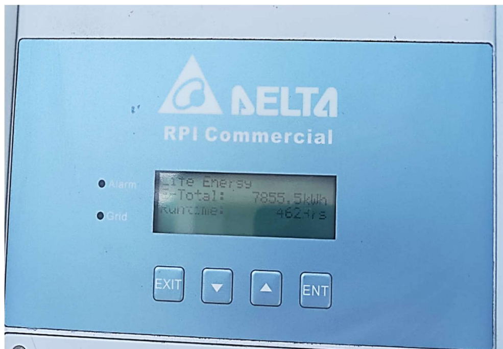
Data taken from solar inverter- (Monthly energy log in kWh)
